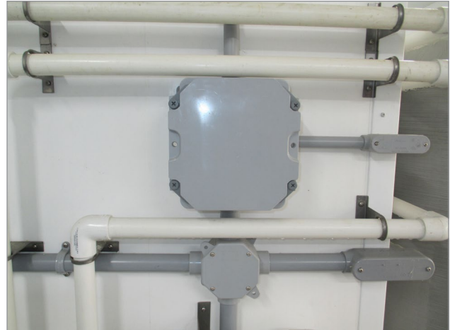
Figure 10. NEMA 4X rated enclosure. Source: Heartland Farm Mutual, Waterloo, Ontario.
