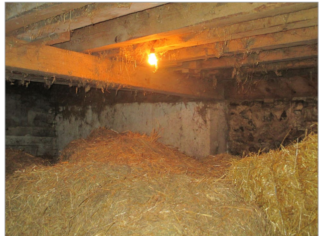
Figure 13. Flammable material near light fixture. Source: Heartland Farm Mutual, Waterloo, Ontario.
