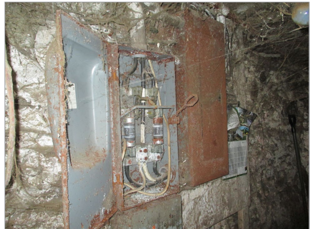
Figure 4. Corroded disconnect panel. Source: Heartland Farm Mutual, Waterloo, Ontario.
