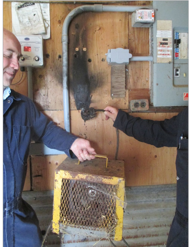
Figure 11. Fire started at box heater with receptacle and plug. Source: Heartland Farm Mutual, Waterloo, Ontario
