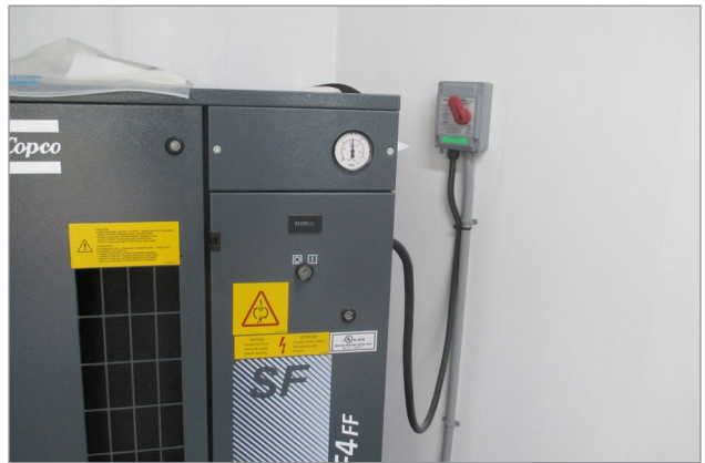
Figure 8. Hard-wired compressor. Source: Heartland Farm Mutual, Waterloo, Ontario
