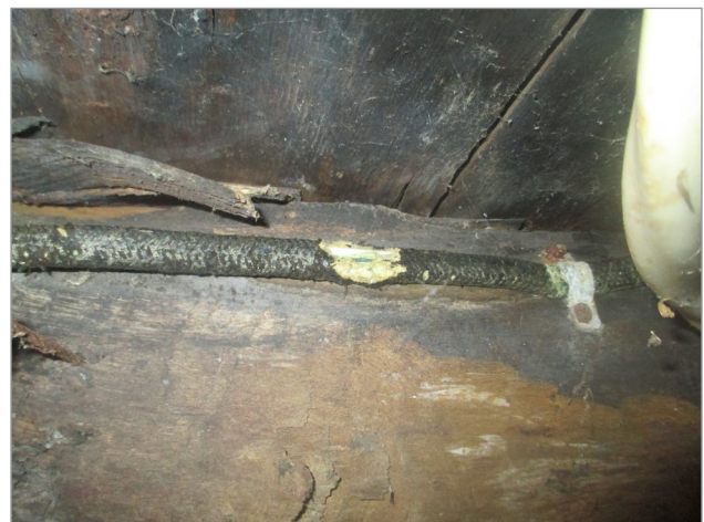
Figure 5. Rodent damage on electrical cable. Source: Heartland Farm Mutual, Waterloo, Ontario.
