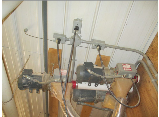
Figure 7. Common plugs and receptacles are not recommended for use in barn environments. Source: Heartland Farm Mutual, Waterloo, Ontario.
