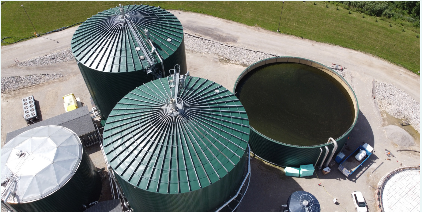
Biogas Digesters at StormFisher's London Biogas Facility.
