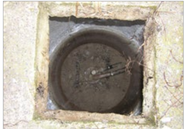
Figure 7. An existing well pit created by constructing a drilled well in an old large-diameter well.
