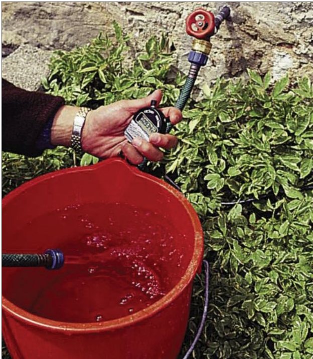
Figure 5. Timing how long it takes for the pump to fill a bucket of water.
