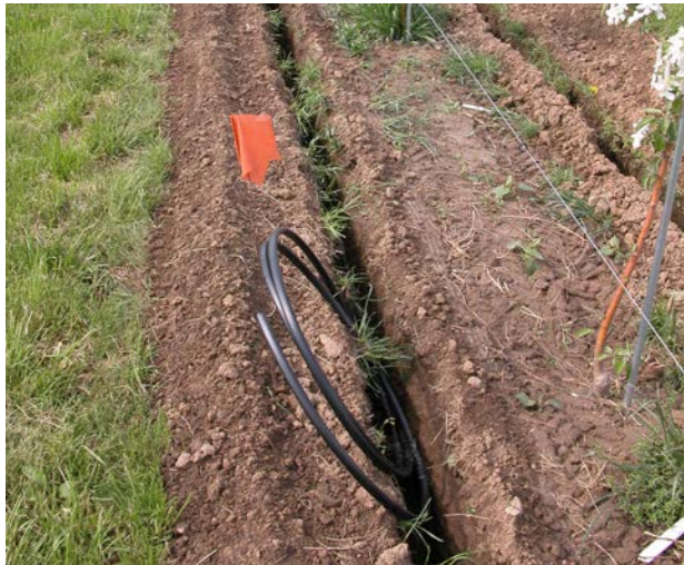
Figure 3-8. Two drip irrigation lines being buried along each side of a row of young fruit trees.
