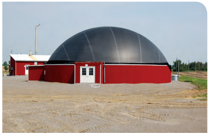
Figure 37. Raised base of liquid storage with tightly-sealed inflatable dome cover visible (V6).
