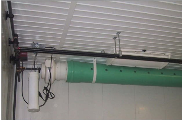
Figure 3. Air circulation assist using a rigid duct with fan and air distribution holes.
