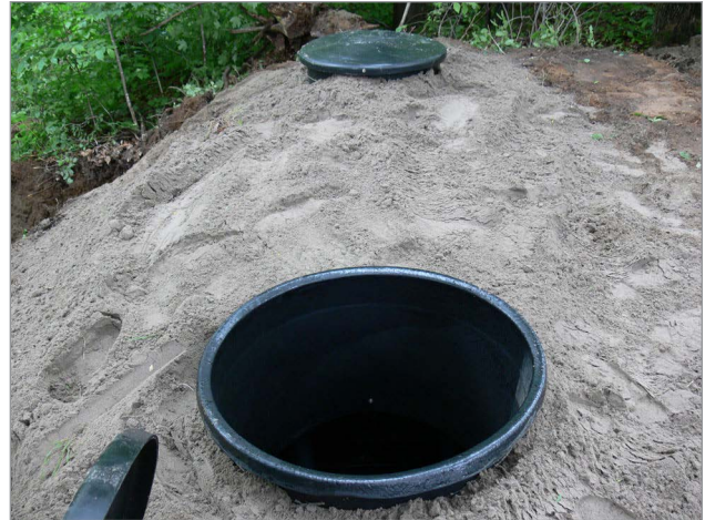
Figure 5. This newly installed, horizontally oriented disposal vessel, made of recycled plastic by an Ontario manufacturer, is easy to transport and install. Two holes facilitate uniform filling. Sandy soil has been added around the vessel for larvae to find a convenient place to pupate.
