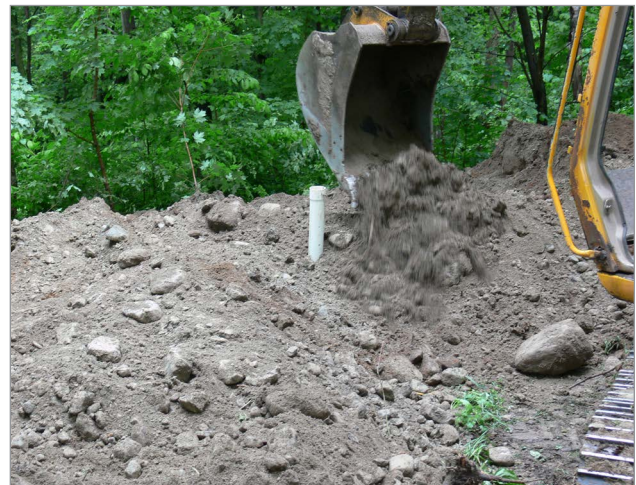
Figure 9. Use the soil from excavating the hole for a new vessel to decommission a vessel that is full. An experienced excavator can do the job in a few hours, with proper planning.
