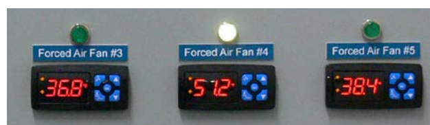
Figure 6. Controller/monitoring equipment associated with Figure 4 FAC system.
