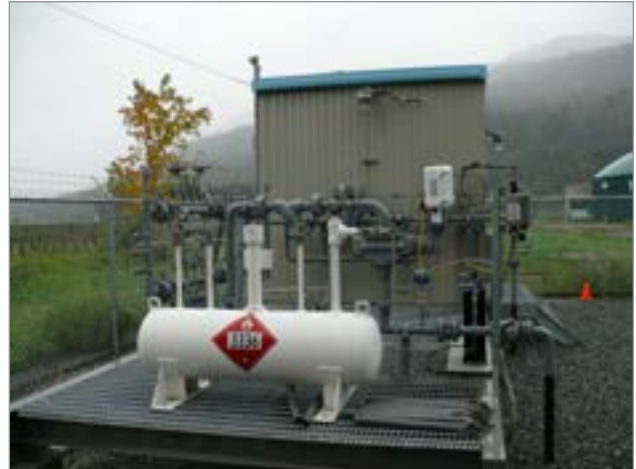
Figure 2. Injection system used to pump RNG into a natural gas line at a farm-based biogas system.
