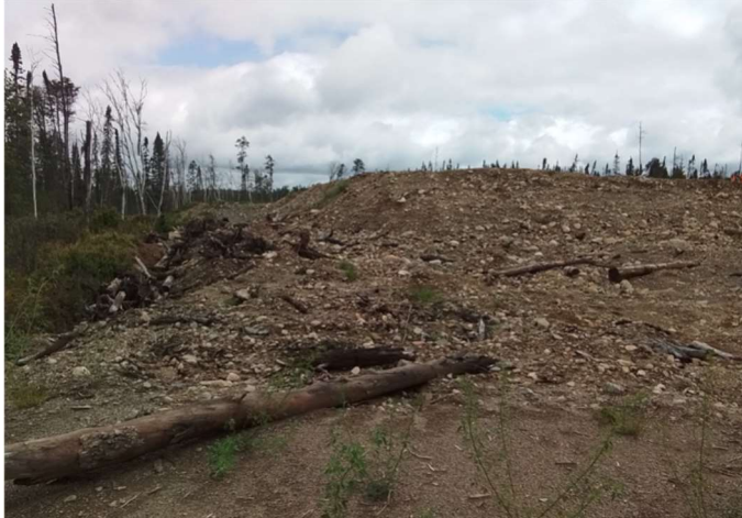
Figure 9. Aggregate pit with steep embankment
